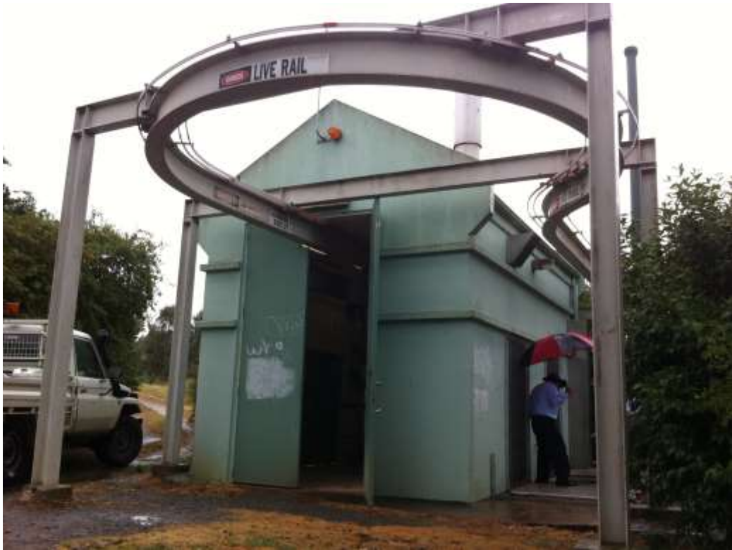
Photo 4.1 River Bank SPS
