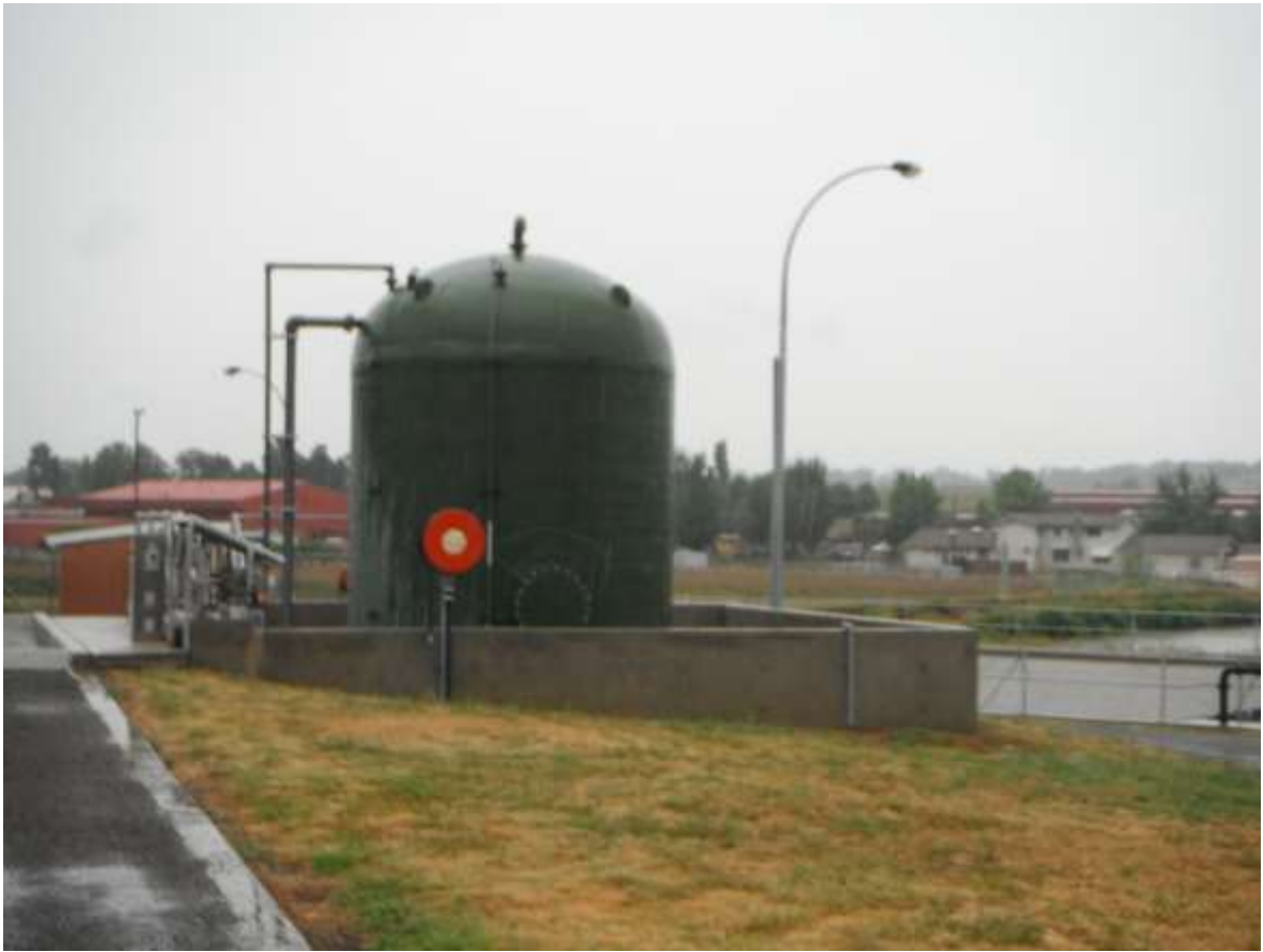
Figure 4.5 STP - Alum Storage Tank, Bund and Delivery Area Bund
