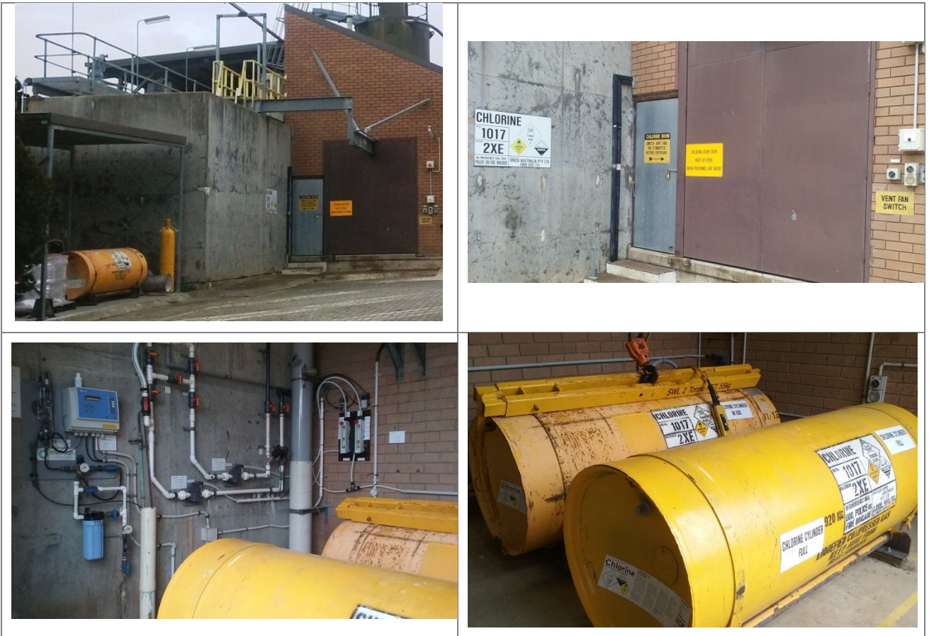
Photo 4.4 Chlorine Gas Storage and Dosing Area
