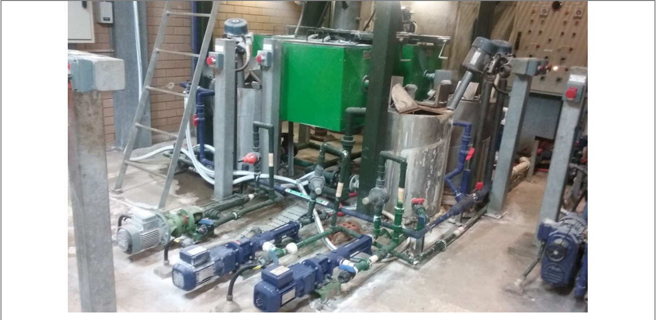
Photo 4.3 Soda Ash Storage and Dosing Area
