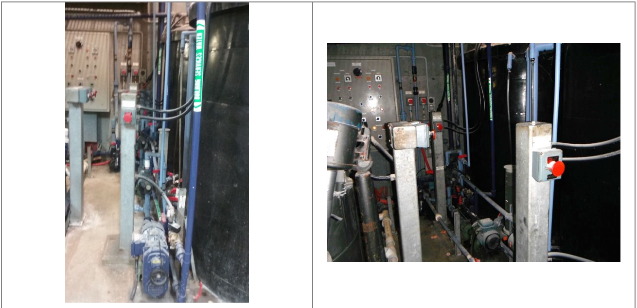
Photo 4.2 Polymer Dosing Area
