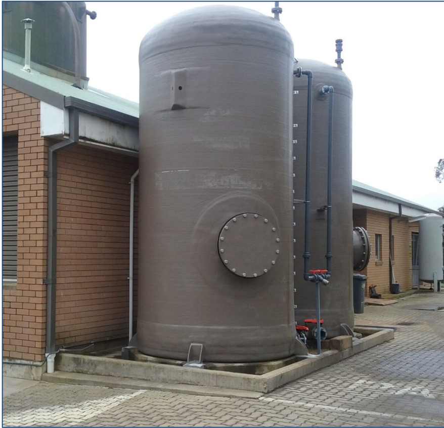
Photo 4.1 Alum Storage Tanks
