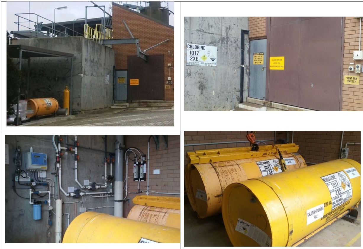
Photo 4.4 Chlorine Gas Storage and Dosing Area
