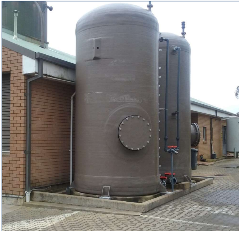
Photo 4.1 Alum Storage Tanks
