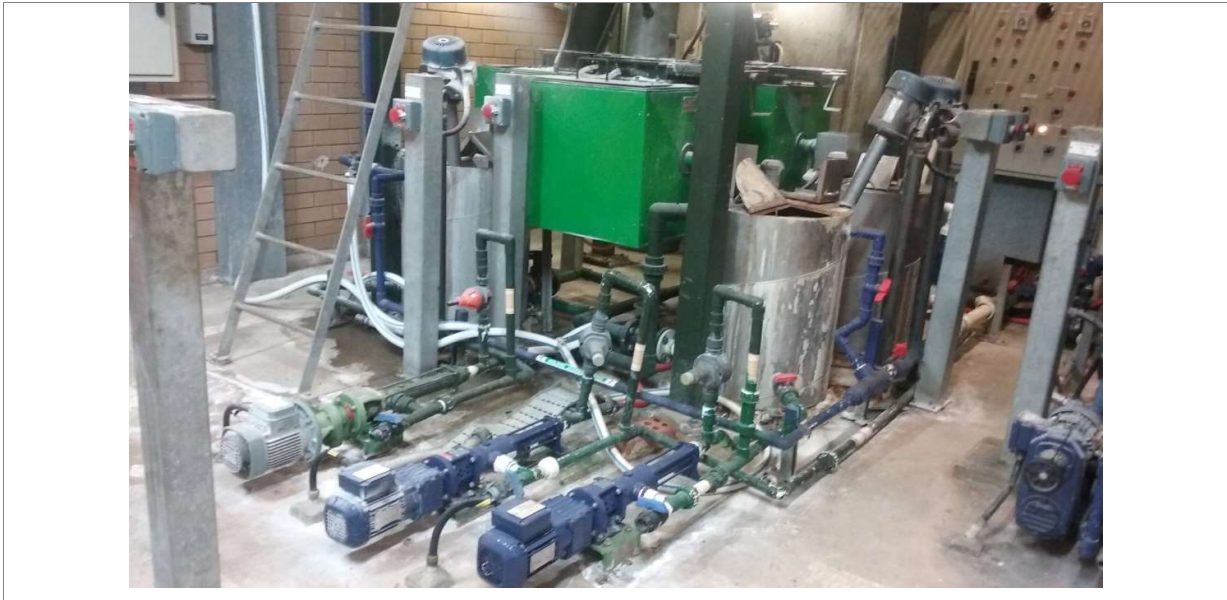
Photo 4.3 Soda Ash Storage and Dosing Area
